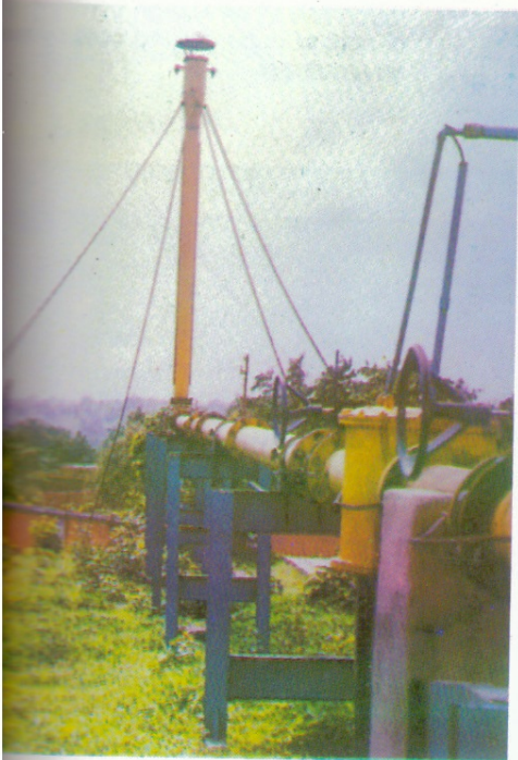
Riser pipe and drain pipe assembly, Amlabad, BCCL
