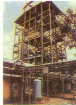
A view of Moving bed Pressure Coal gasification plant
