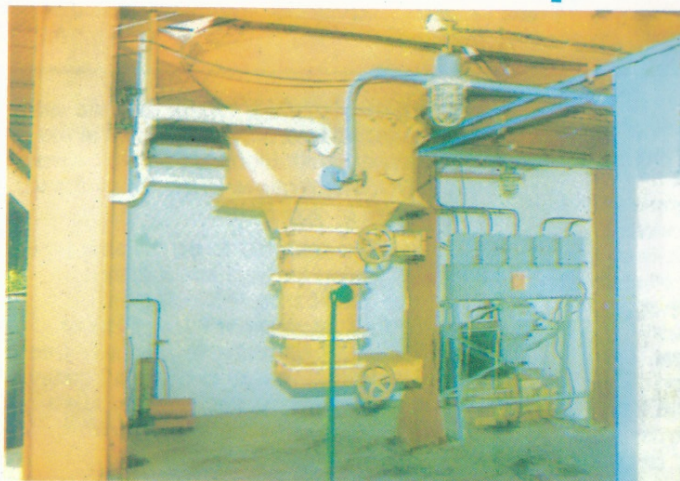
Ash Discharge Arrangement, Fluidised Bed Gasifier
