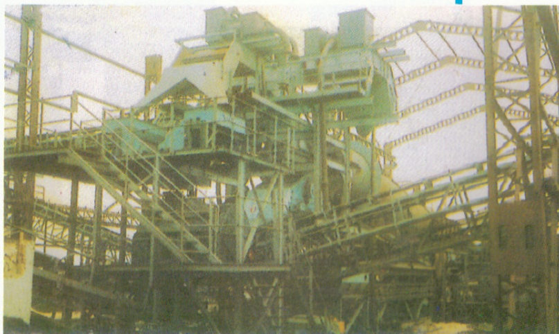
Close-up of pilot plant incorporating barrel washer
